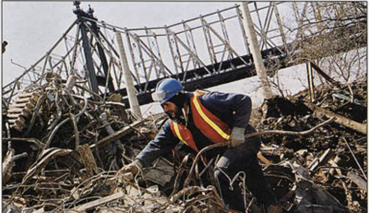
"A shot in the arm" – A Laborer sifts through the debris on the Roosevelt Island project, which is in full swing.
